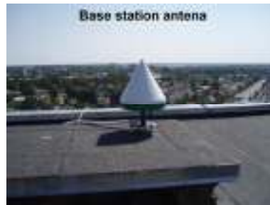
Fig. 7. Base station North (Kre)
